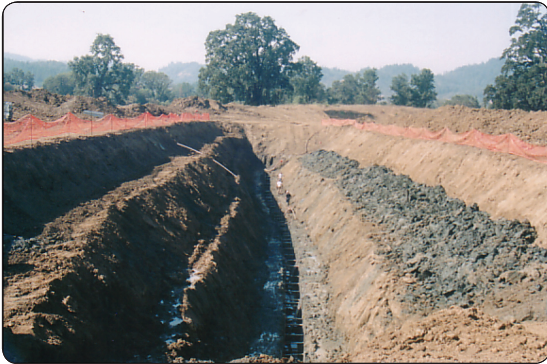
Figure 4. Overview of one of the deep trench excavations for the Frank R. Howard Memorial hospital fault rupture hazard investigation. Holocene alluvial sediments are present in the sidewalls above the floor of the pit; late Pleistocene “lacustrine” sediments are below the pit floor, in the walls of the shored trench. Note the gleyed, gray-colored “lacustrine” spoils on the mid-pit bench, which contrast with the oxidized yellow-brown Holocene alluvial soils.
